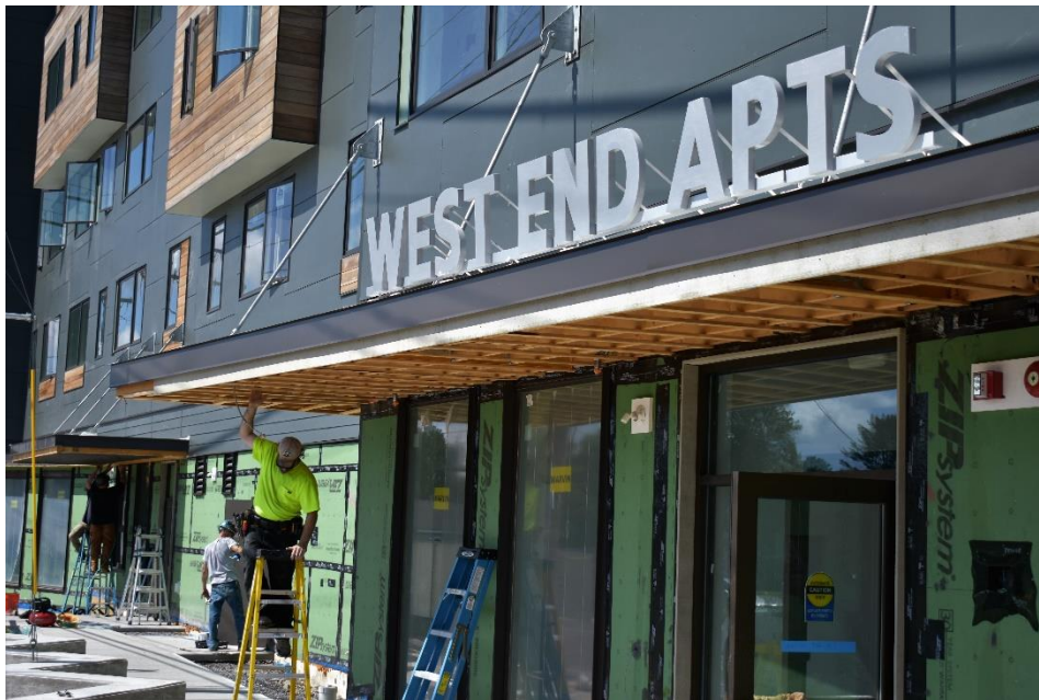
Above: Workers wrap up construction of 52 permanent housing units at West End II in South Portland. (Photo credit: Avesta Housing)
