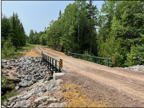
A folding steel temporary bridge installed at the Eagle Lake Unit, BPL Northern Region. The bridge addressed a barrier to fish passage at this stream crossing and improved access to a significant amount of upstream trout habitat.
